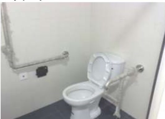
Figure. 17 WC for PWDs with grab rails (SSS)
